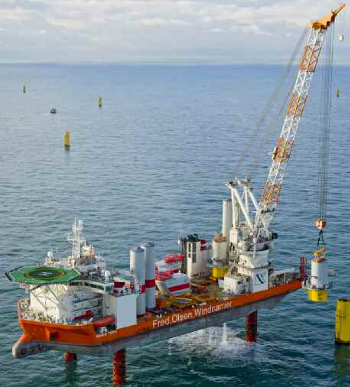
February 11, 2014 – In the beginning of 2014 the self-elevating wind turbine installation vessel Brave Tern owned by Fred. Olsen Windcarrier was operating in the Global Tech 1 Offshore Wind Park for the installation of wind turbines.
