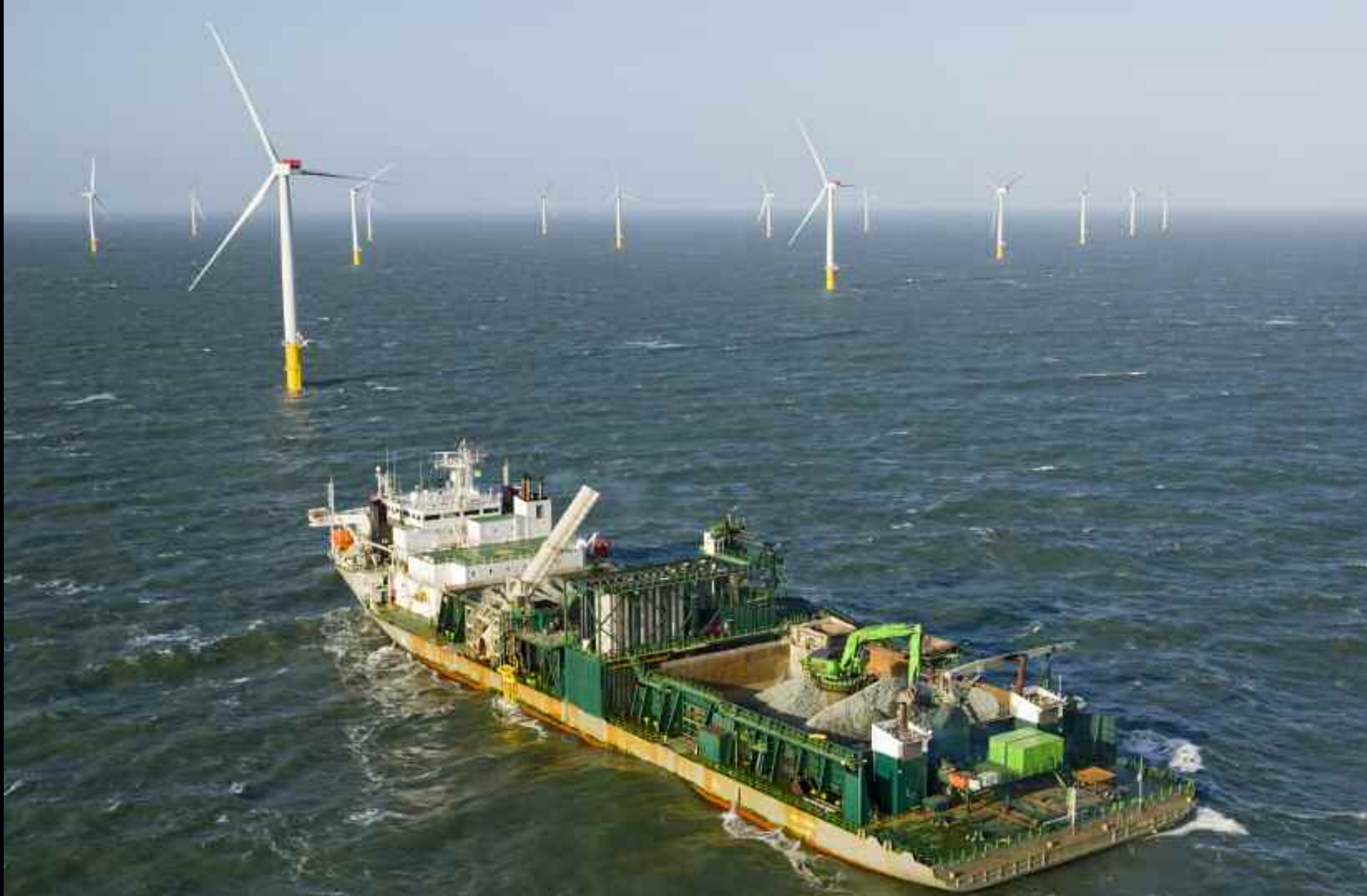
January 24, 2015 – Also the fallpipe vessel Seahorse has been deployed for scour protection work in the Gwynt y Mor area.
