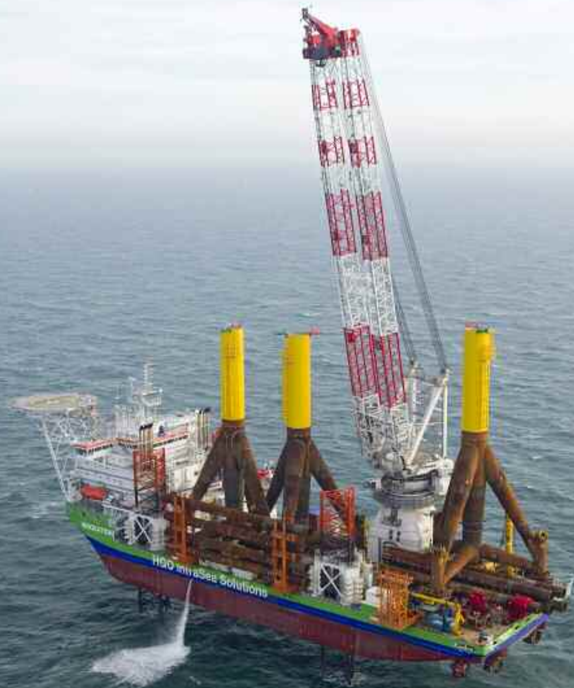
October 22, 2013 – The self-elevating wind turbine installation vessel Innovation operated by HGO Infra Sea Solutions just before starting to use her 1,500-ton Liebherr crane to install the first out of three turbine foundations in the Global Tech 1 Offshore Wind Farm.
