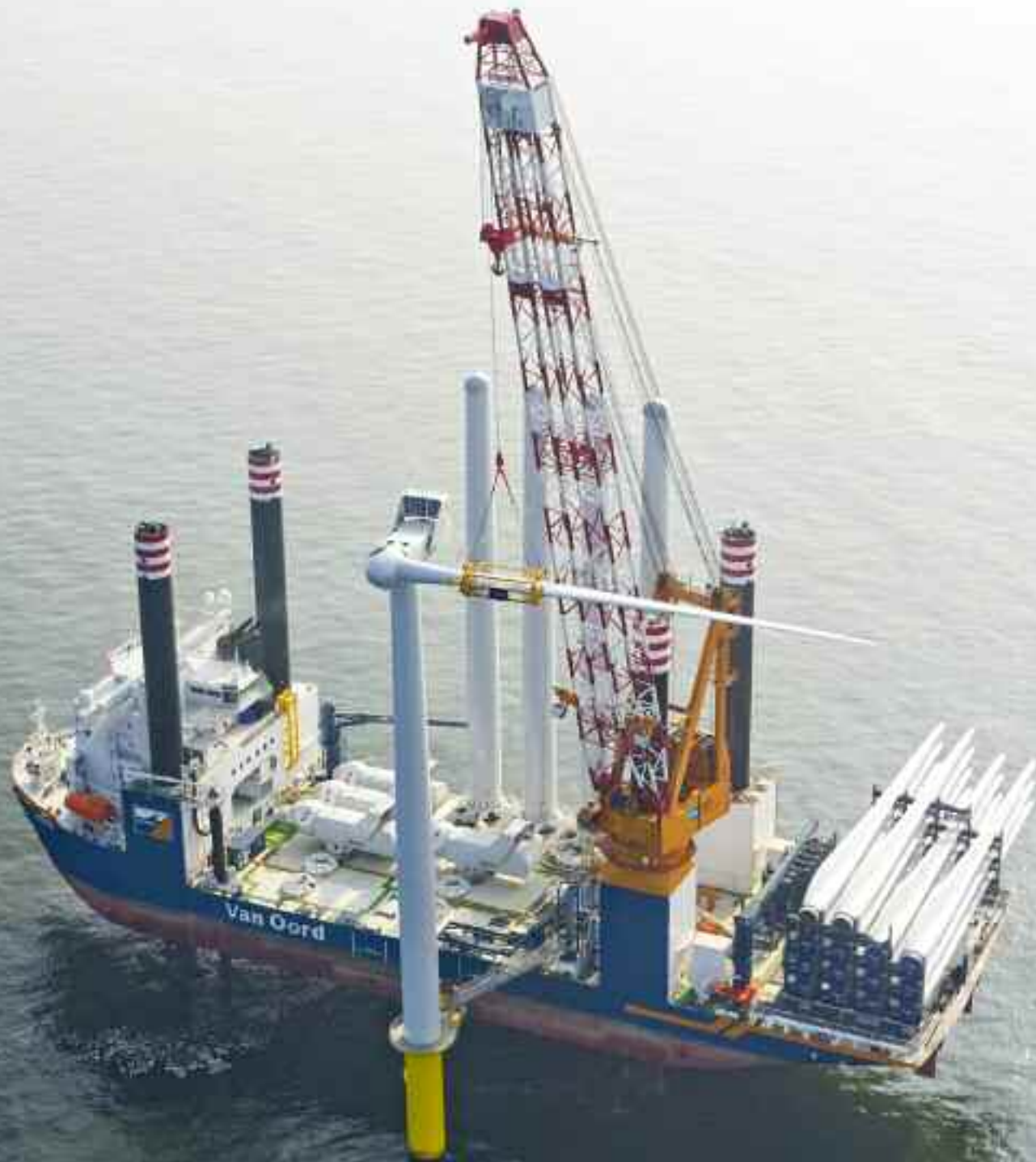
April 9, 2015 – The 139 metre long Aeolus is equipped with a large crane with a lifting capacity of 900 ton to lift towers, nacelles and blades. The vessel can work in water down to 55 metre of depth.
