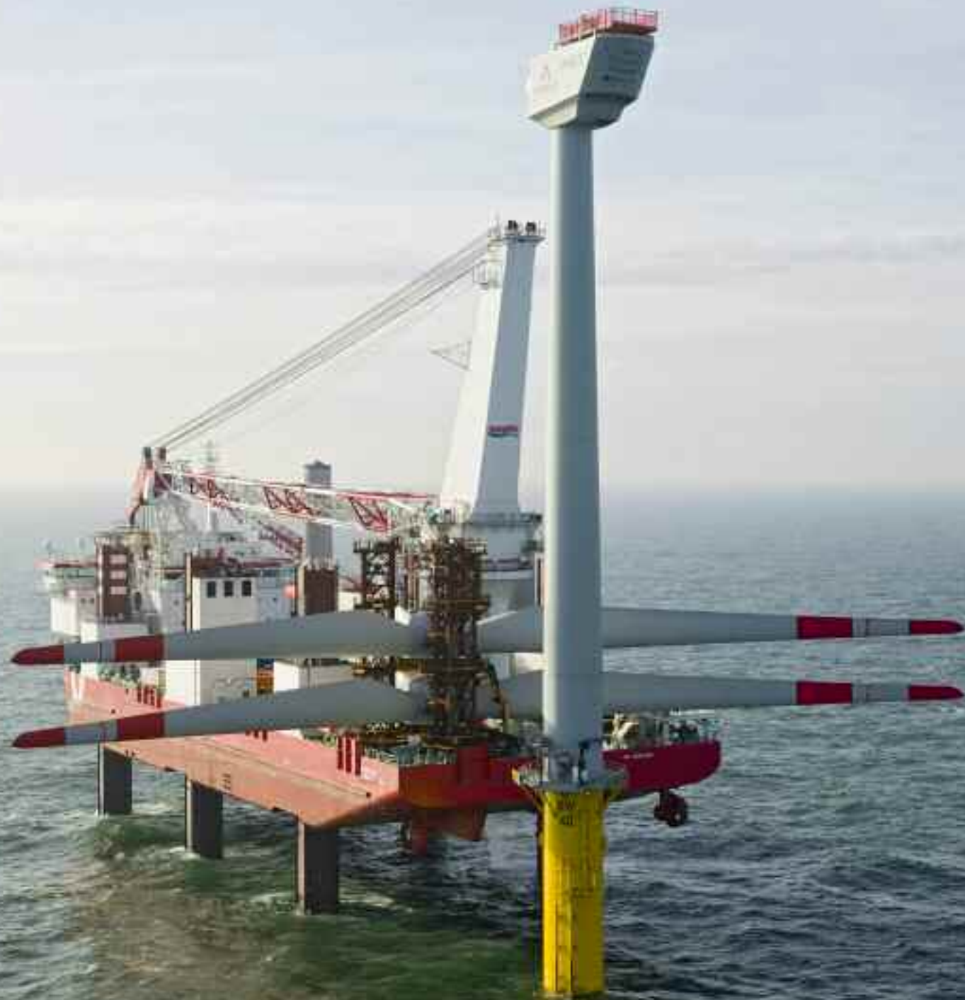
October 22, 2013 – The MPI Adventure owned by MPI Offshore during installation of nacelles and rotors in the Borkum West Offshore Wind Farm.
