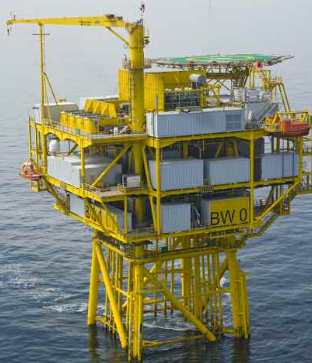
April 29, 2014 – The BW-0 substation is situated 25 Nautical miles north of the German island Borkum in the Borkum West Offshore Wind Farm. The farm includes 80 turbines.
